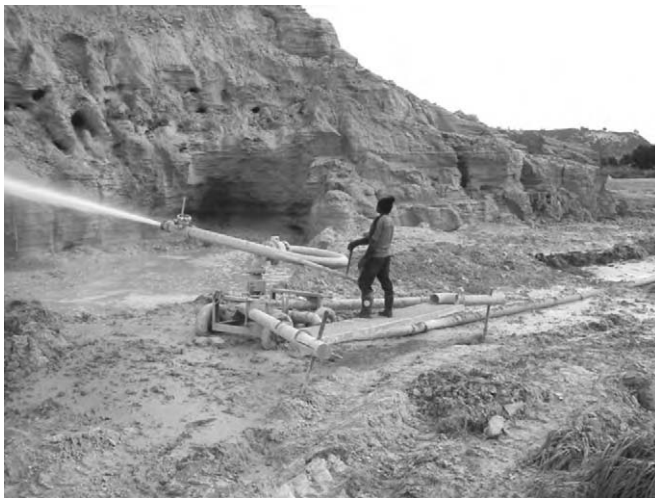
Fig. 3. Manually controlled monitor gun.
