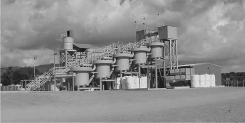
Fig. 5. Five-stage carbon adsorption column plant (CIC plant) built by Kappes, Cassidy & Associates for Glamis Gold's San Martin, Honduras project. There are two parallel column trains (one is behind the other in this view). The plant can process up to 900\text{ m}^3 of solution per hour, and is sized for an operation that processes up to 20,000 tonnes of ore per day.
