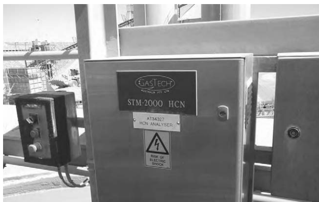
Fig. 4. On-line HCN gas analyser at SDGM CIL section.
