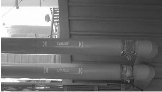
Fig. 6. Cyanide pipe colour coding and flange guards.
