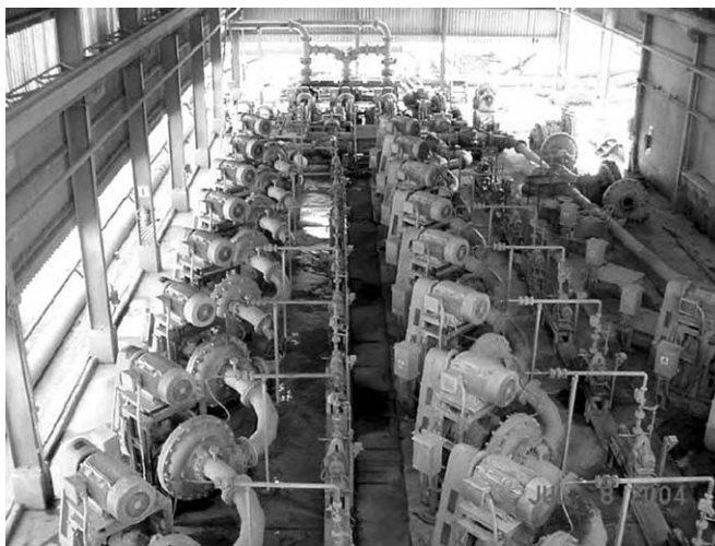
Fig. 5. Main transfer pump-station.
