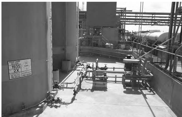
Fig. 7. Liquid cyanide storage tank and bund.
